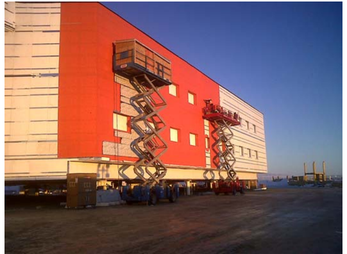
Over 65,000 sq. ft of WrapShield SA Self-Adhered was installed at Norton Sounds.
